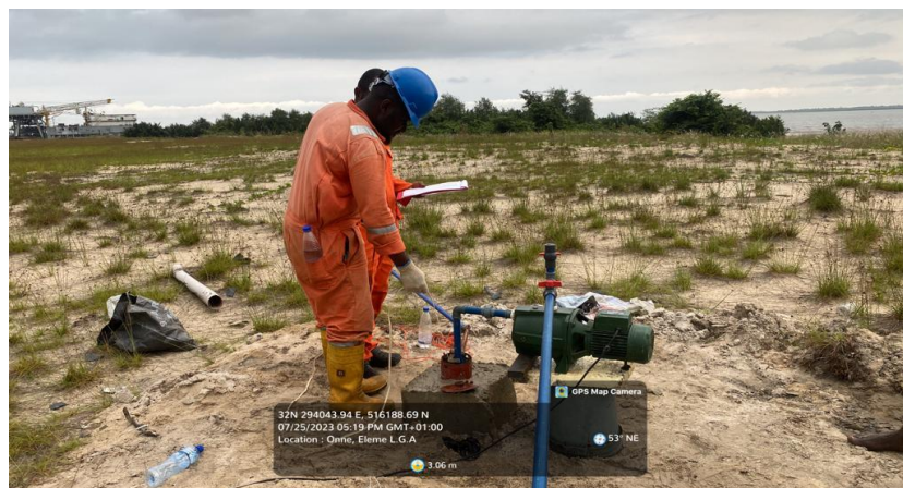
Figure 2.8: Hydraulic conductivity determination using a surface pump and a data logger installed in the borehole
