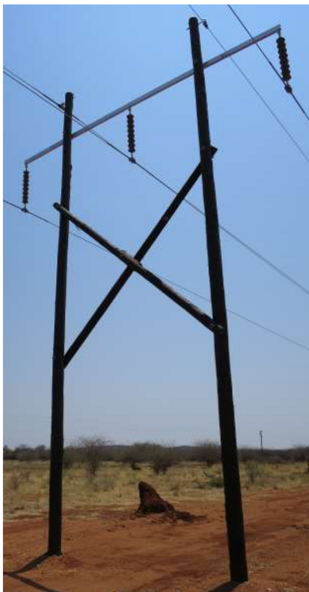
Plate 2.1: Example of the 66kV wooden structure with wooden crossarm (Source: Transmission Consulting Services (TCS), 2020).
