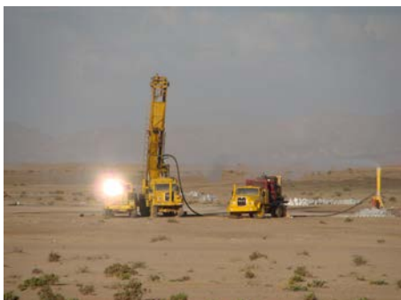
LEFT: Drilling in progress on the central Namib gravel plains. This is an archaeologically sensitive surface and detailed survey should precede drilling.
