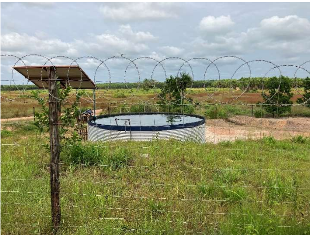
Plate 2-11: Fire water station tank within plantation area Sierra Leone
