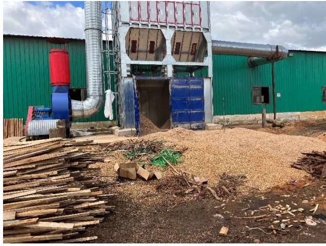
Plate 2-6: Dust extraction / dry waste segregation Sierra Leone
